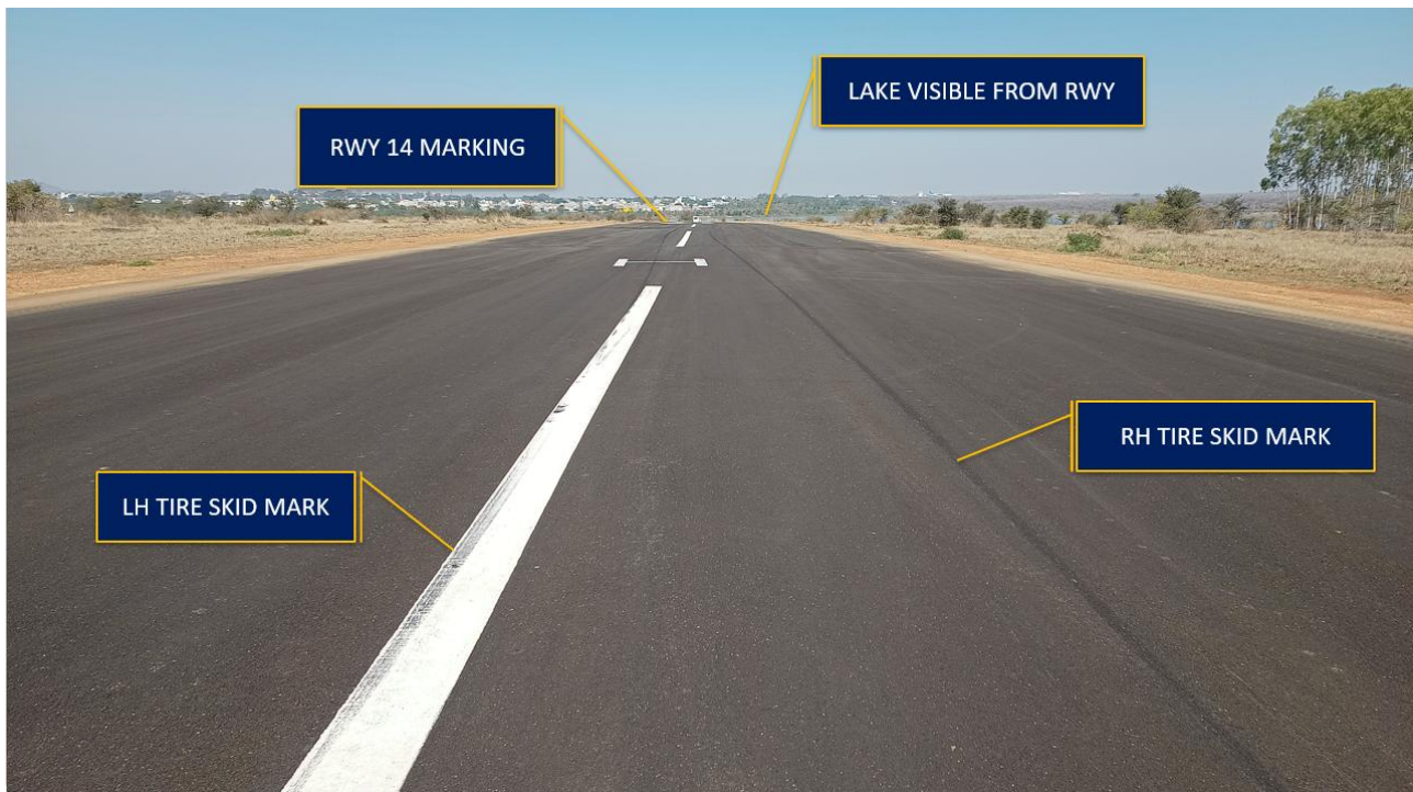
Figure 4. Tire Skid Marks
